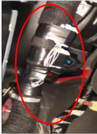
Connector is covered by tape with wiring. Carefully cut the tape to release the connector/harness.
